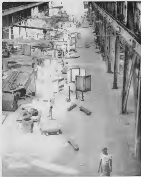
Pipe, boiler, and welding shops (4, 5) are being temporarily set up in this building which used to hold the machining shop. Pipe bending machine will be located in left foreground (notice pit in floor); a 4,500 sq. ft. welding shop space (8) will be added to side at left.
